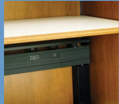
J-Channel manages and distributes electrical and data.
